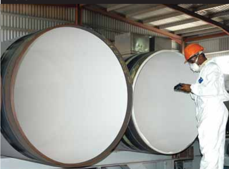
▼ Pipes protected with WaterGuard® LE
