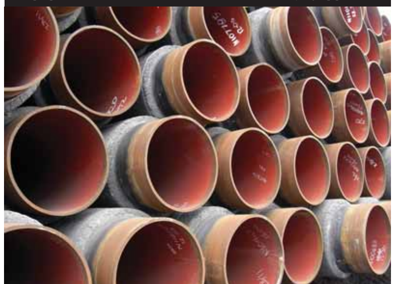
▼ Pipes protected with SureFlo® SF which will be installed for the Gjøa gas pipeline
